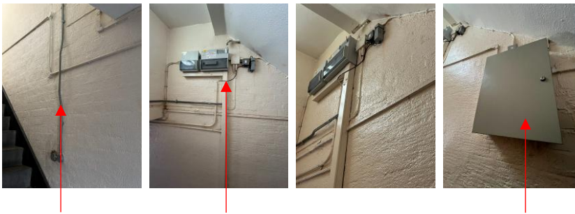
Metal conduit, metal enclosed D.B, metal Door access control power supply.
