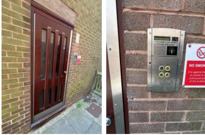
Entrance with door access control to the block
