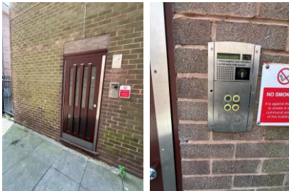
Entrance door access systems.
