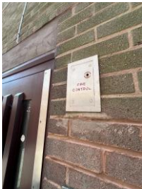
Firefighter's switches at only the front entrance
