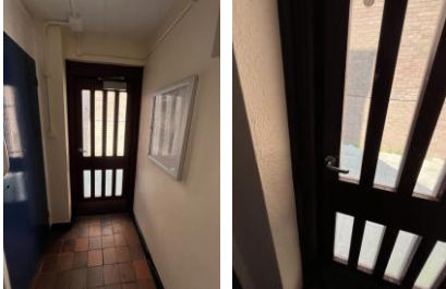
Final exit door and levered handle
