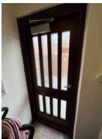
Final exit door and levered handle
