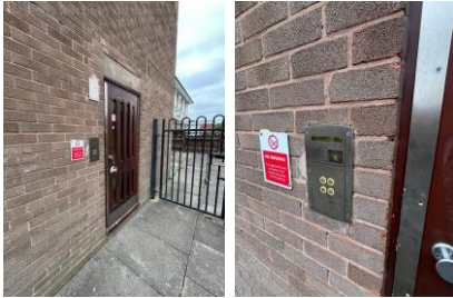
Entrance door access systems.
