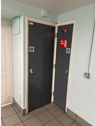
Dry riser cupboard
