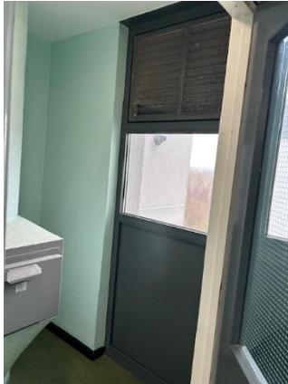
Vented bin chute
