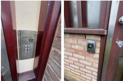
Both entrance door access systems.
