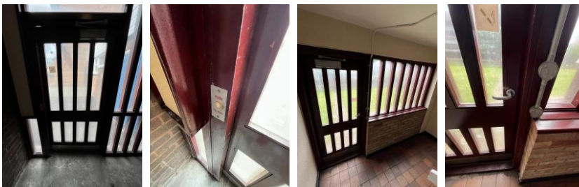
Final exit doors and doors exits buttons
