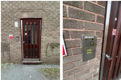
Entrance door access systems.
