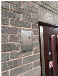
Firefighter's switches at only the front entrance
