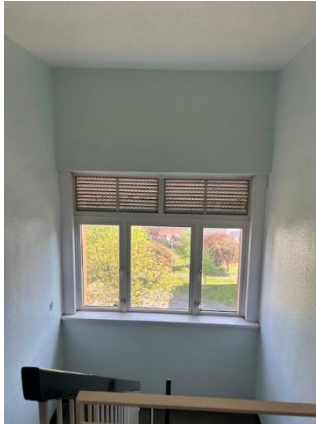
Manual window and fixed vent to protected staircase
