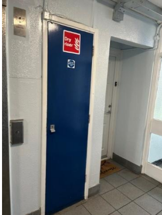
Dry riser inlet cupboard
