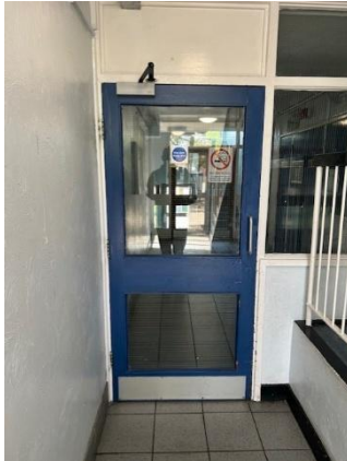
Common area fire door
