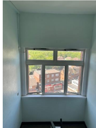
AOV window to protected staircase
