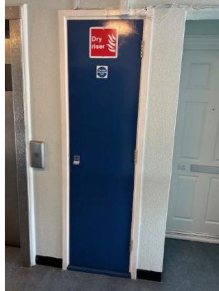
Dry riser outlet cupboard
