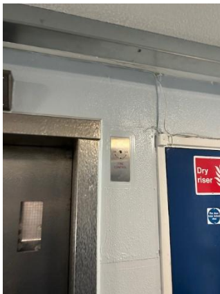
Firefighting control switch
