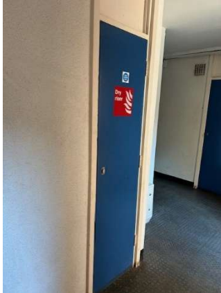
Dry riser inlet cupboard
