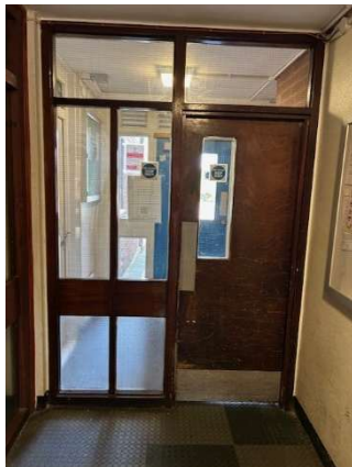
Common area fire door
