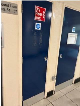
Dry riser cupboard
