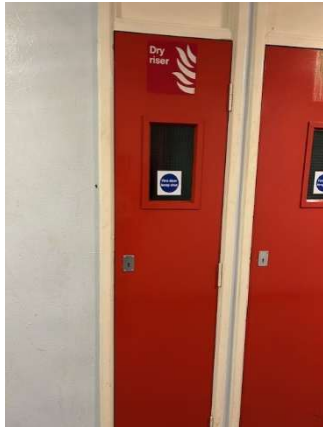
Dry riser outlets – all levels
