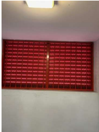
Louvre vent (15 th floor)
