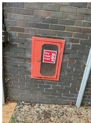
Dry riser inlet
