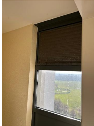
Fixed vent to bin chute
