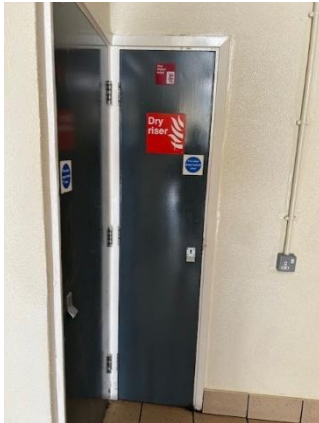
Dry riser cupboard
