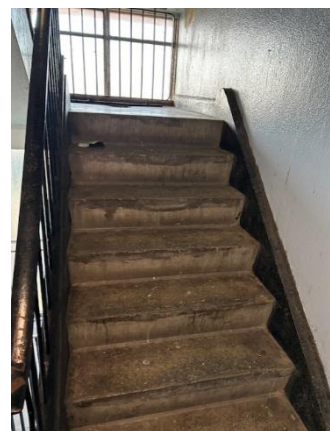
Staircase to 14 th floor plant rooms
