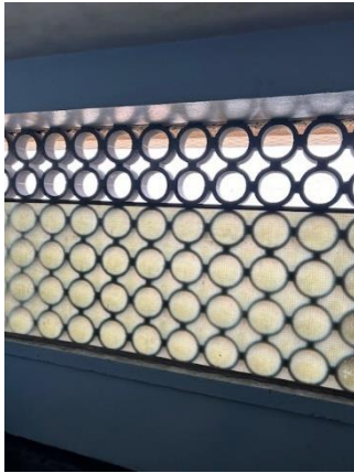
Fixed vent to bin chute
