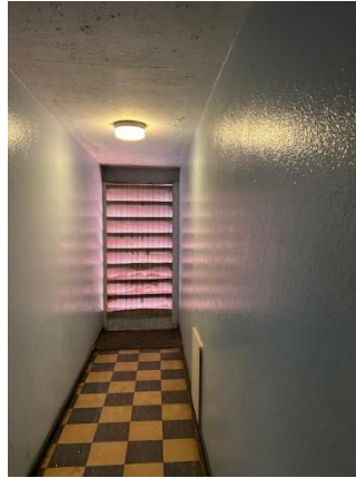
Fixed vent to corridor
