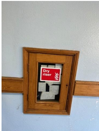
Dry riser inlet
