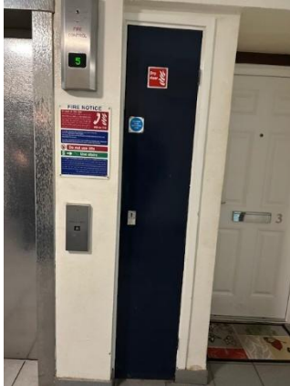
Dry riser inlet cupboard
