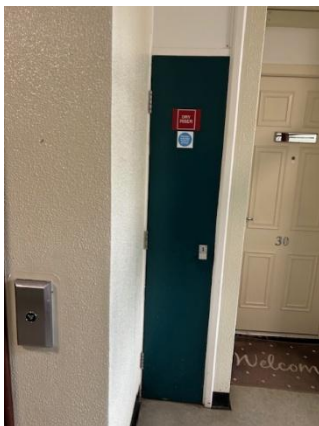
Dry riser outlet cupboard
