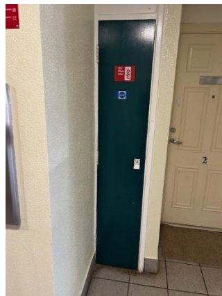
Dry riser inlet cupboard
