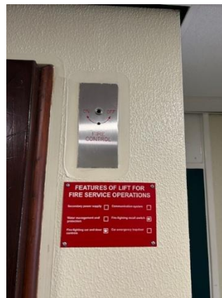
Lift informational Firefighter control switch
