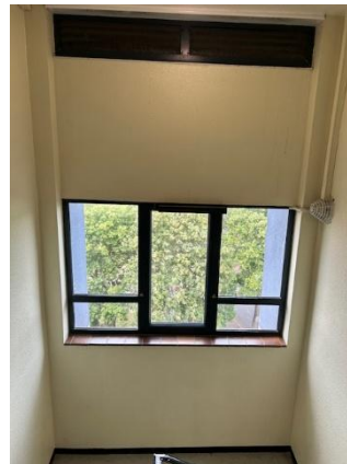
AOV window to staircase
