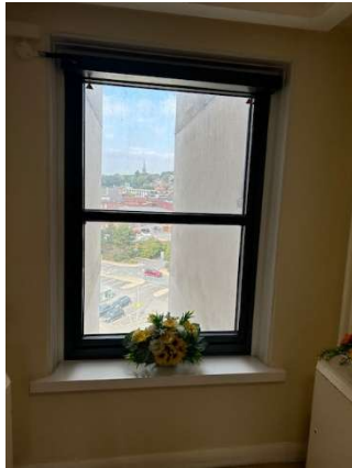
AOV window to flat corridor
