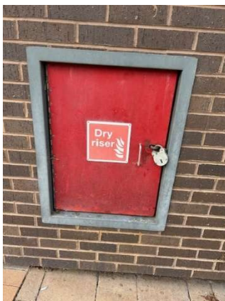
Dry riser inlet
