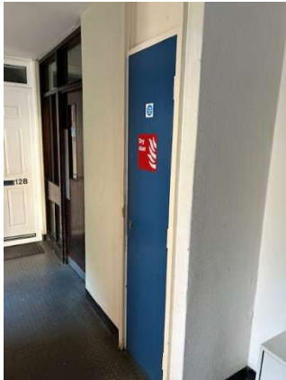
Dry riser outlet cupboard
