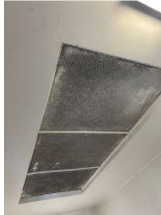
Ventilation grill (5 th floor)
