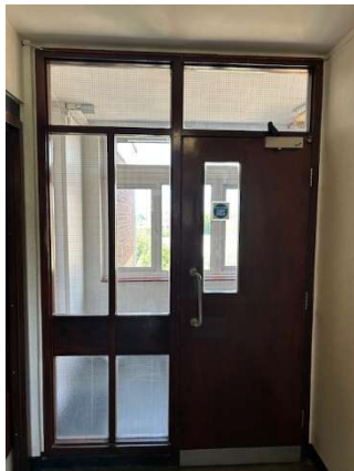
Common area fire door
