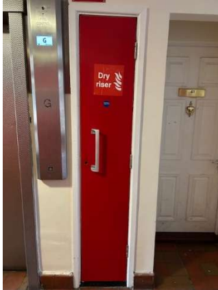
Dry riser inlet cupboard
