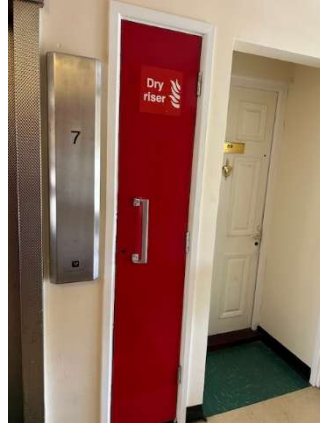
Dry riser outlet cupboard
