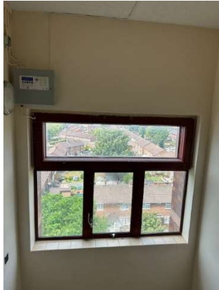
AOV window to staircase
