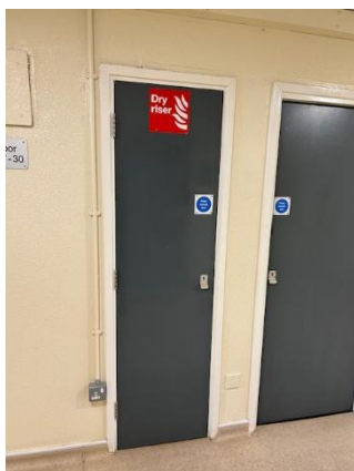
Dry riser outlet cupboard
