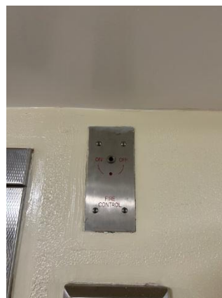
Firefighting control switch
