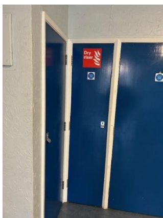
Dry riser cupboard
