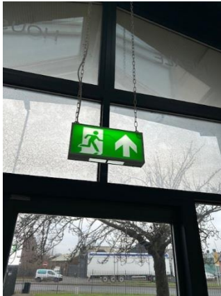
Bulkhead directional signage above final exit
