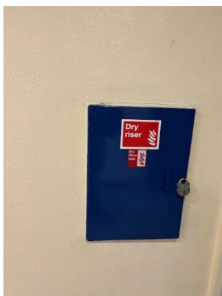
Dry riser inlet
