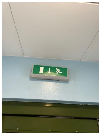
Bulkhead directional emergency lighting
