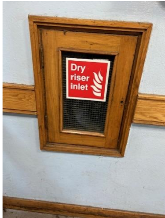
Dry riser inlet
