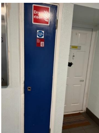
Dry riser inlet cupboard
