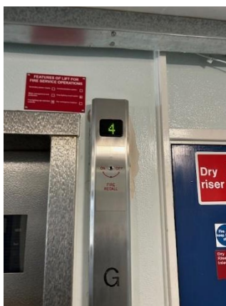
Firefighting control switch
