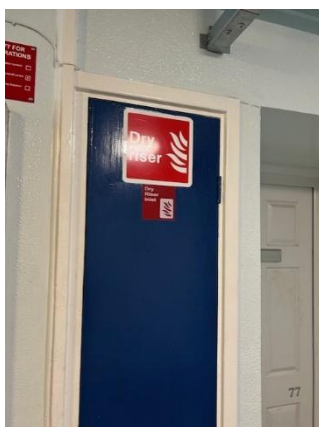
Dry riser inlet cupboard
