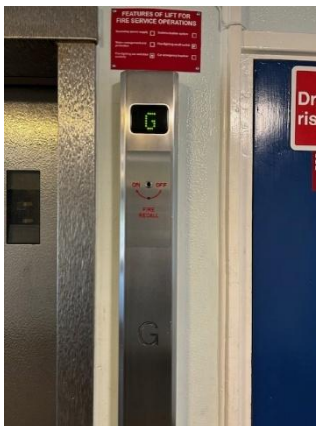
Firefighters lift switch
