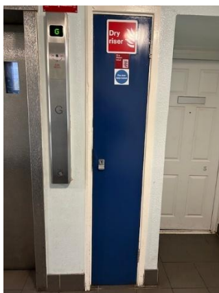
Dry riser cupboard
