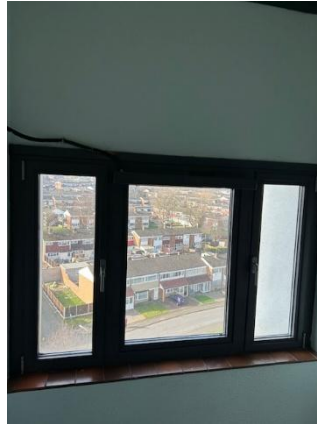
AOV window (8 th floor front staircase)
