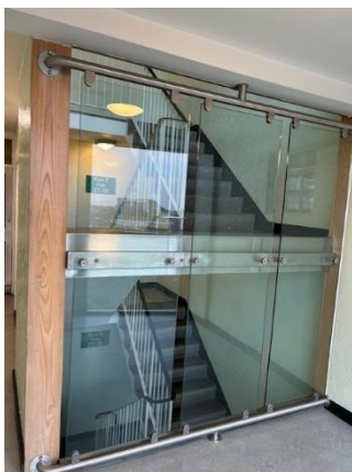
Gaps between glass to staircase on the 7th floor
