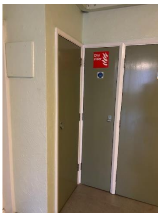
Dry riser cupboard
