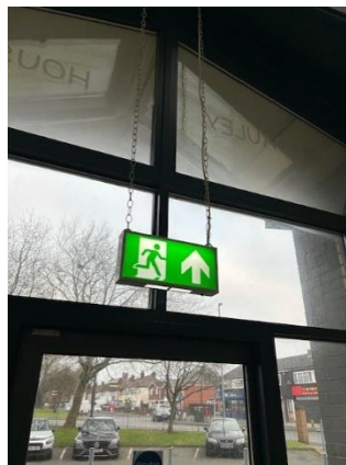
Bulkhead directional signage above final exit
