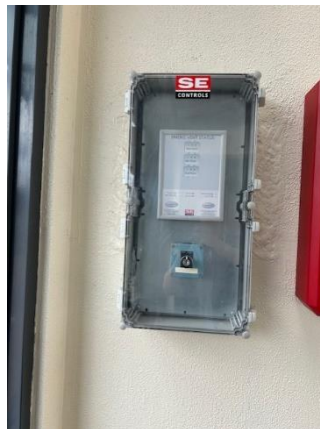
Smoke vent for floors 2, 9 and 16
