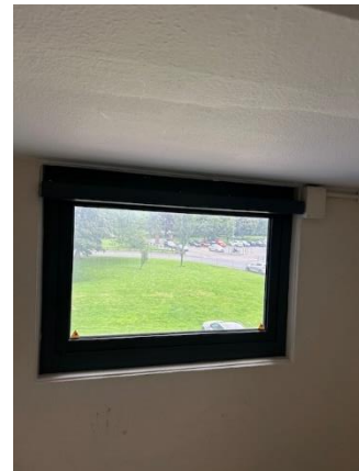
AOV window (stairs, floors 2, 9 and 16)
