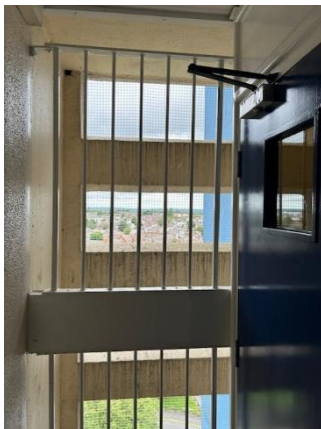
Open vent for lobby
