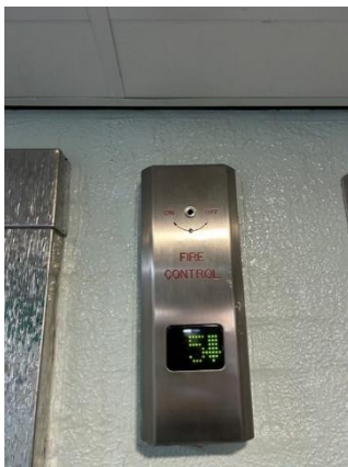
Firefighters control switch
