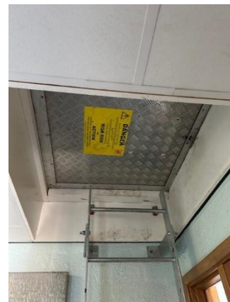
Hatch to lift motor room
