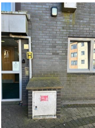
Dry riser inlet
