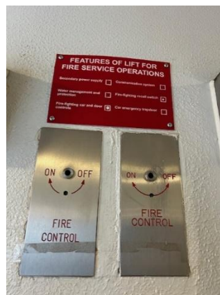
Lift control switches
