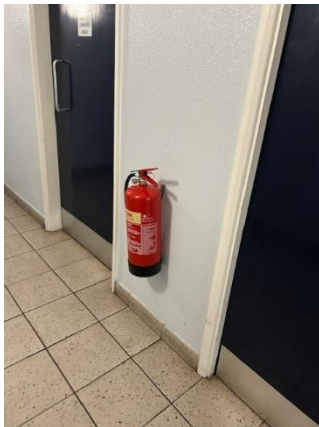
AFFF in basement
