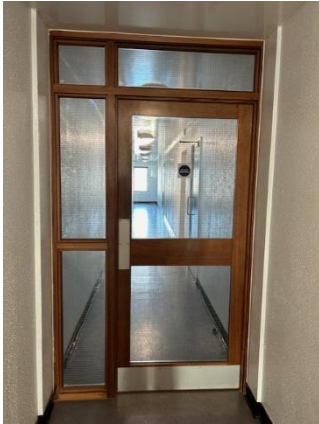
Cross-corridor fire doors
