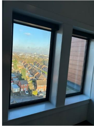
AOV window to staircase
