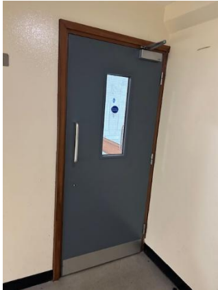
Fire door to single staircase
