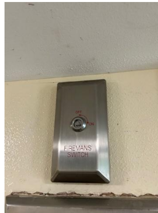
Firefighting control switch
