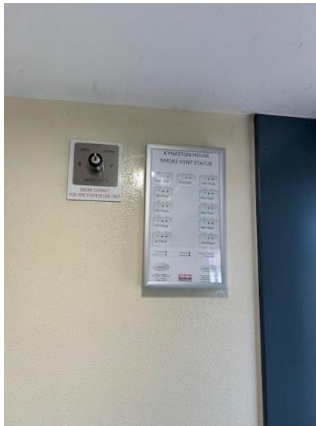
AOV status panel & control switch
