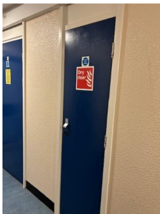
Dry riser all levels
