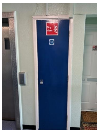
Dry riser outlet cupboard
