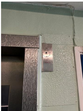
Firefighting control switch
