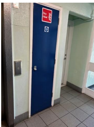
Dry riser inlet cupboard
