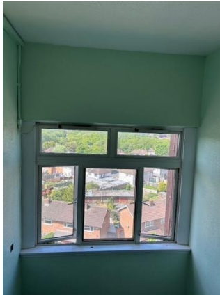
AOV window (7 th floor staircase)
