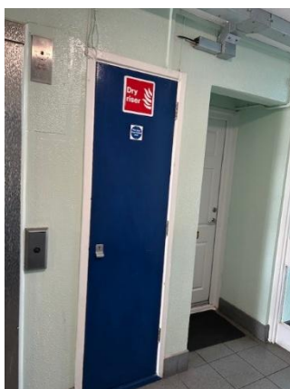
Dry riser inlet
