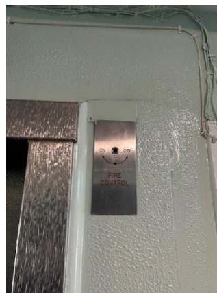
Firefighter control switch
