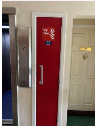
Dry riser outlet cupboard
