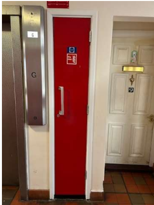
Dry riser inlet cupboard
