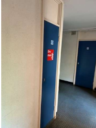
Dry riser inlet cupboard
