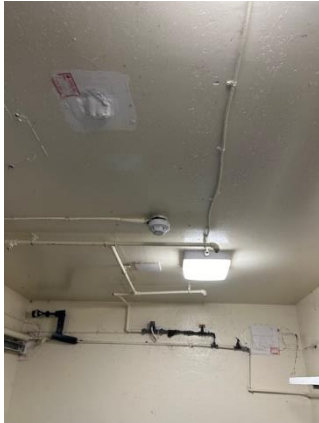
Fire suppression system to bin store
