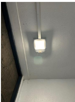
Emergency lighting to staircase
