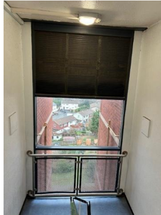
Louvre vent on 10 th floor
