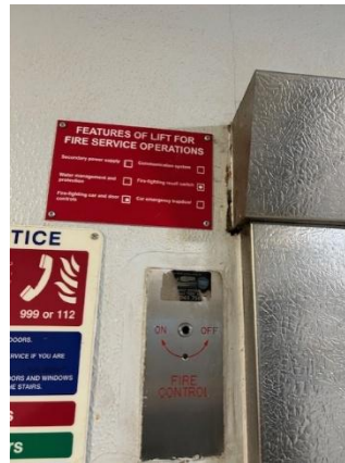
Fire control switch
