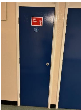
Dry riser outlet in lift lobby
