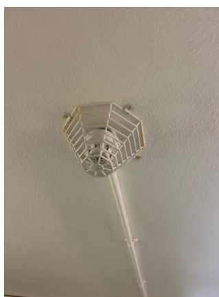
Detection in lift lobby
