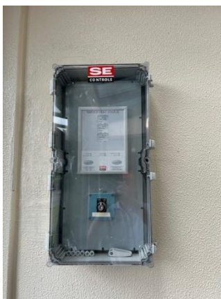
AOV panel in lobby
