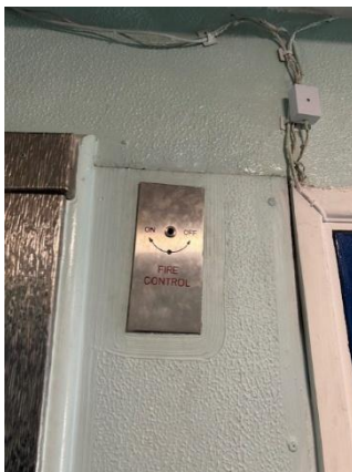
Firefighting control switch
