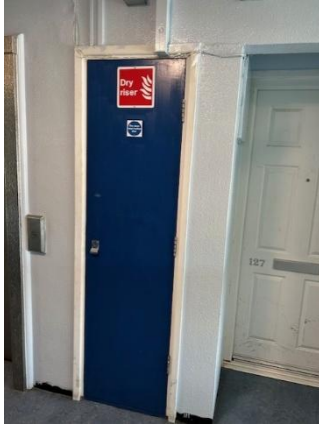
Dry riser outlet cupboard
