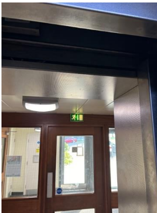
Bulkhead emergency lighting
