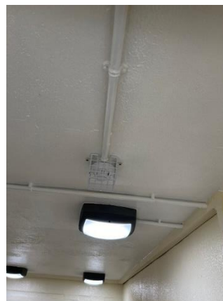
14 th floor stairs detection
