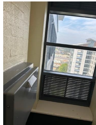
Bin chute ventilation
