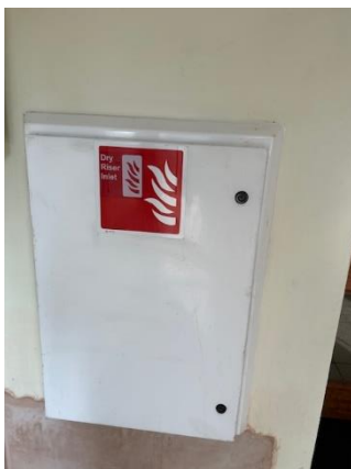
Dry riser inlet
