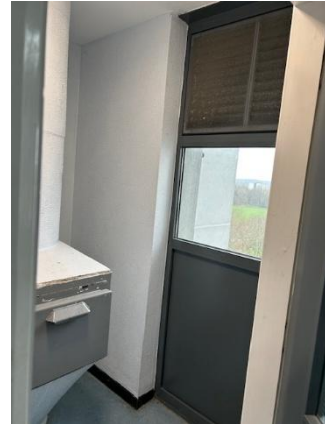
Naturally vented bin chute
