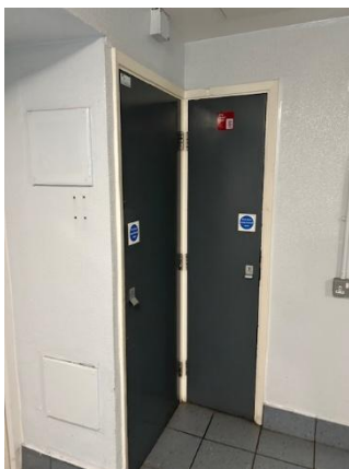
Dry riser inlet cupboard
