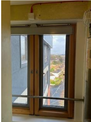
AOV window to lift lobby
