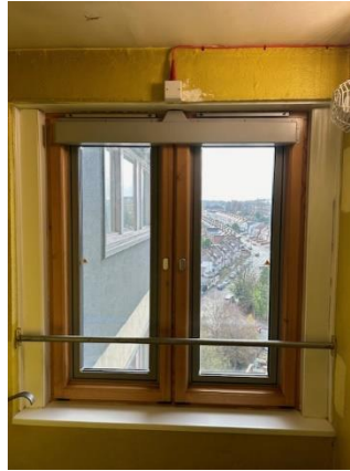
AOV window to staircase
