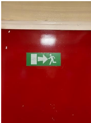
Non-compliant directional signage
