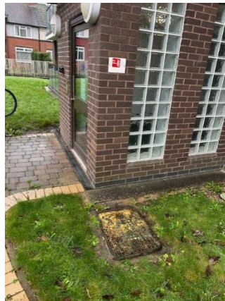
Dry riser inlet
