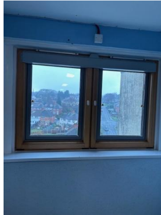
AOV window to lift/flat lobby
