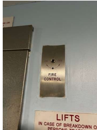
Firefighting control switch
