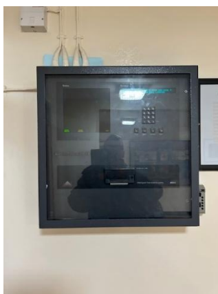
Fire alarm panel
