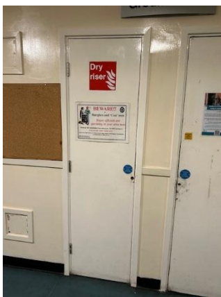
Dry riser cupboard
