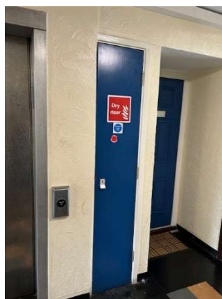
Dry riser outlet cupboard
