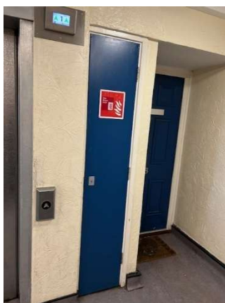
Dry riser inlet cupboard
