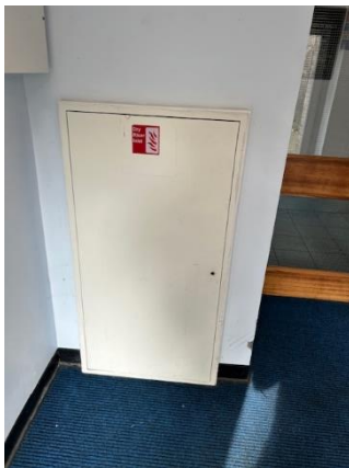
Dry riser inlet
