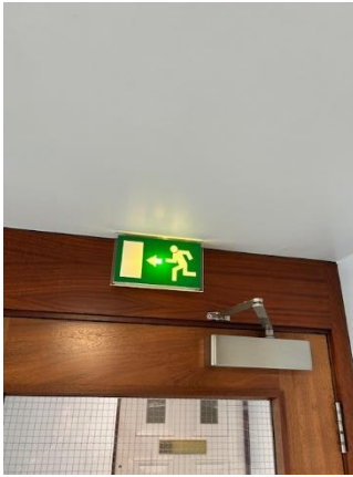
Bulkhead emergency lighting
