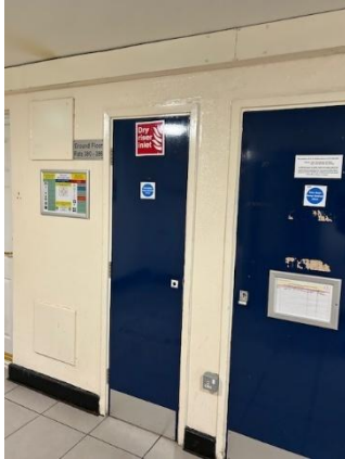
Dry riser inlet
