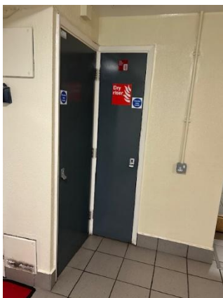
Dry riser cupboard
