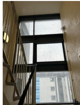
AOV window to staircase
