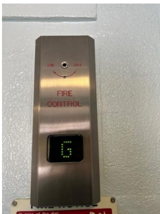
Firefighters control switch
