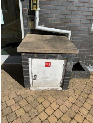
Dry riser inlet
