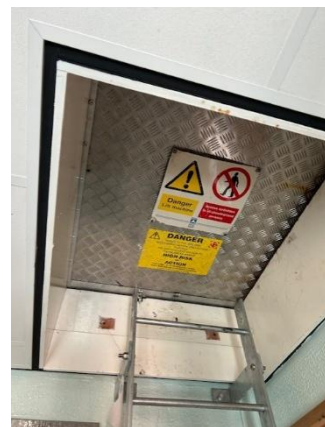
Hatch to lift motor room
