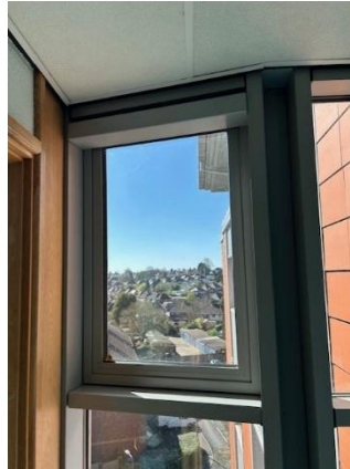
AOV window to staircase
